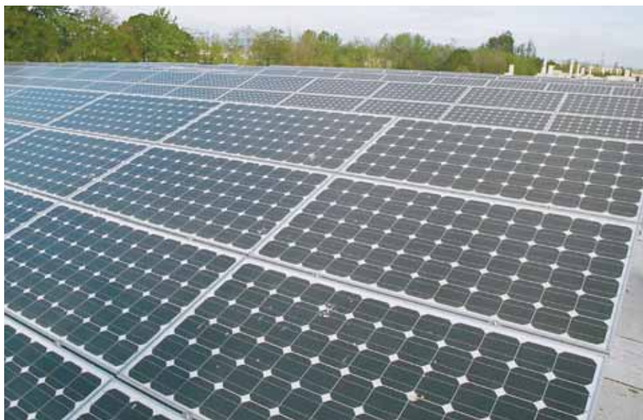
Incentives from the Energy Trust of Oregon as well as Portland General Electric helped put more than 600 solar panels atop Kettle Foods Salem. They provide enough power to make more than 250,000 bags of chips while reducing CO2 emissions by 65 tons. Photo courtesy of Kettle Foods.
